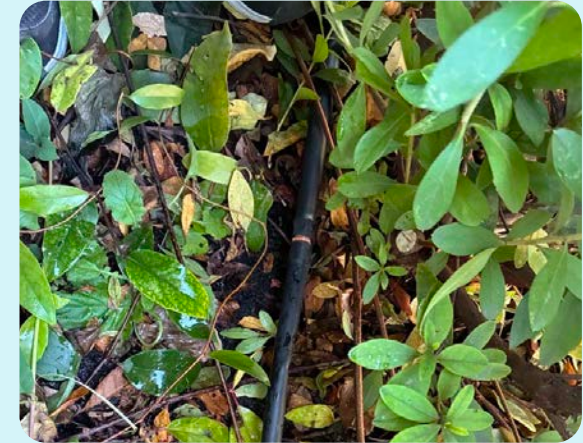
Drip irrigation system supporting efficient landscape watering
