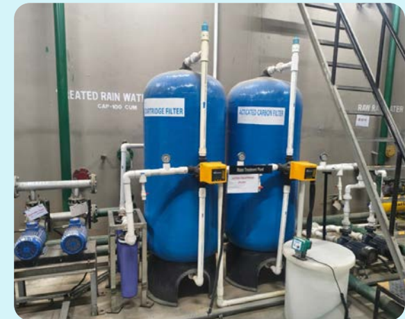
MU1 Water Treatment Plant
